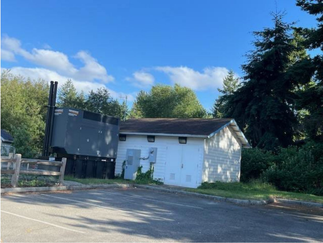
Figure 4. Weathervane Booster Pump Station Emergency Backup Power
