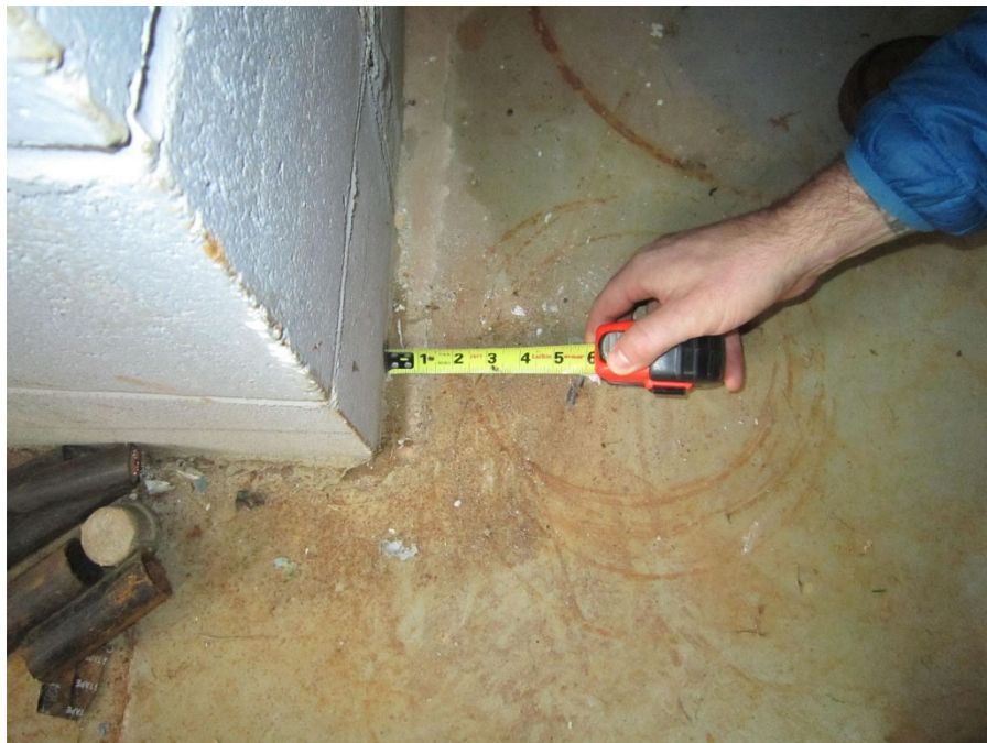
Photo 14 – Control Room Base of Southwest Corner Wall
