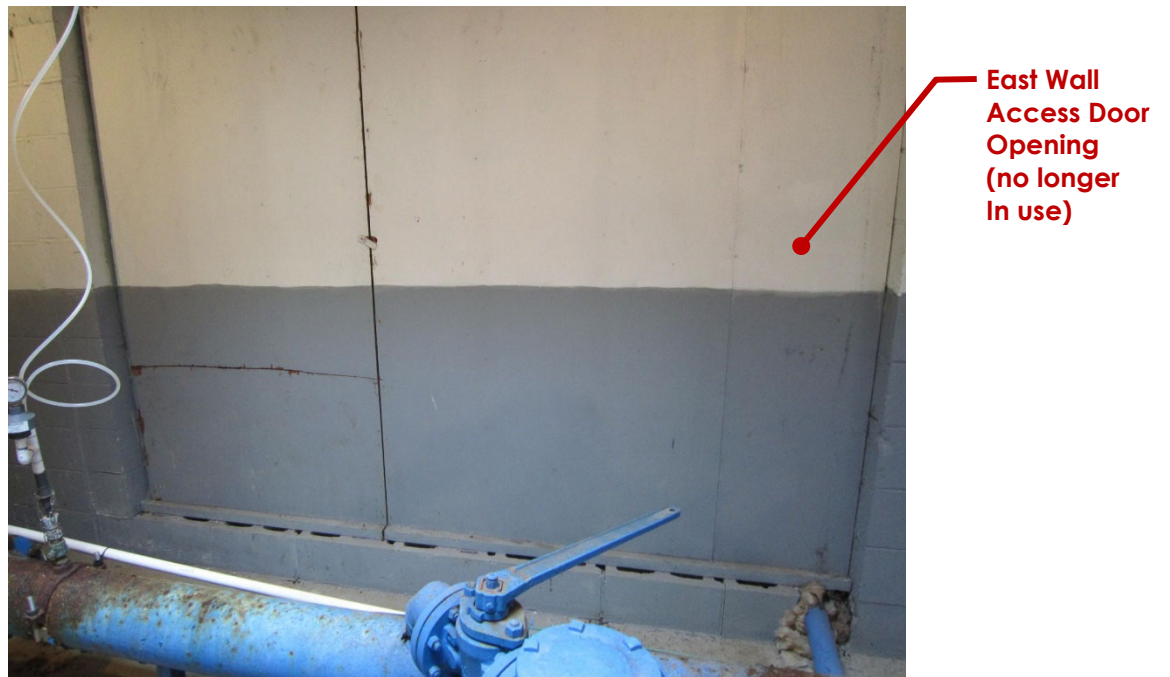
Photo 28 – Flow Meter Room (Looking Northeast)
