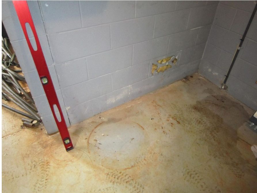
Photo 13 – Control Room Base of Southwest Corner Wall
