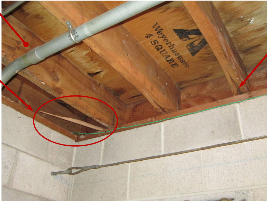
Photo 35 – Old Transformer Room (Looking West)
