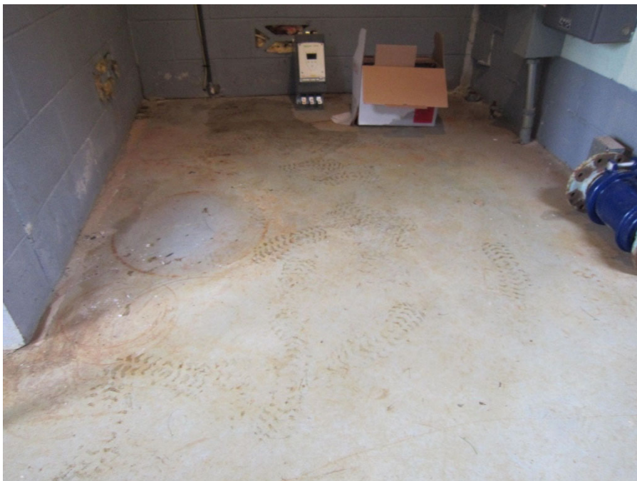
Photo 12 – Control Room (Looking West)
