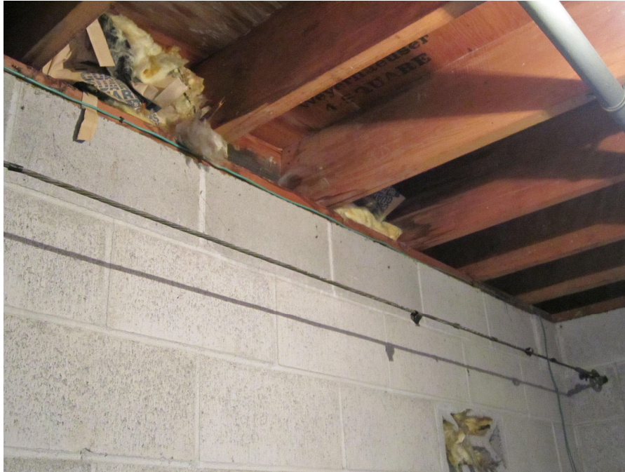
Photo 37 – Old Transformer Room (Looking Northeast)
