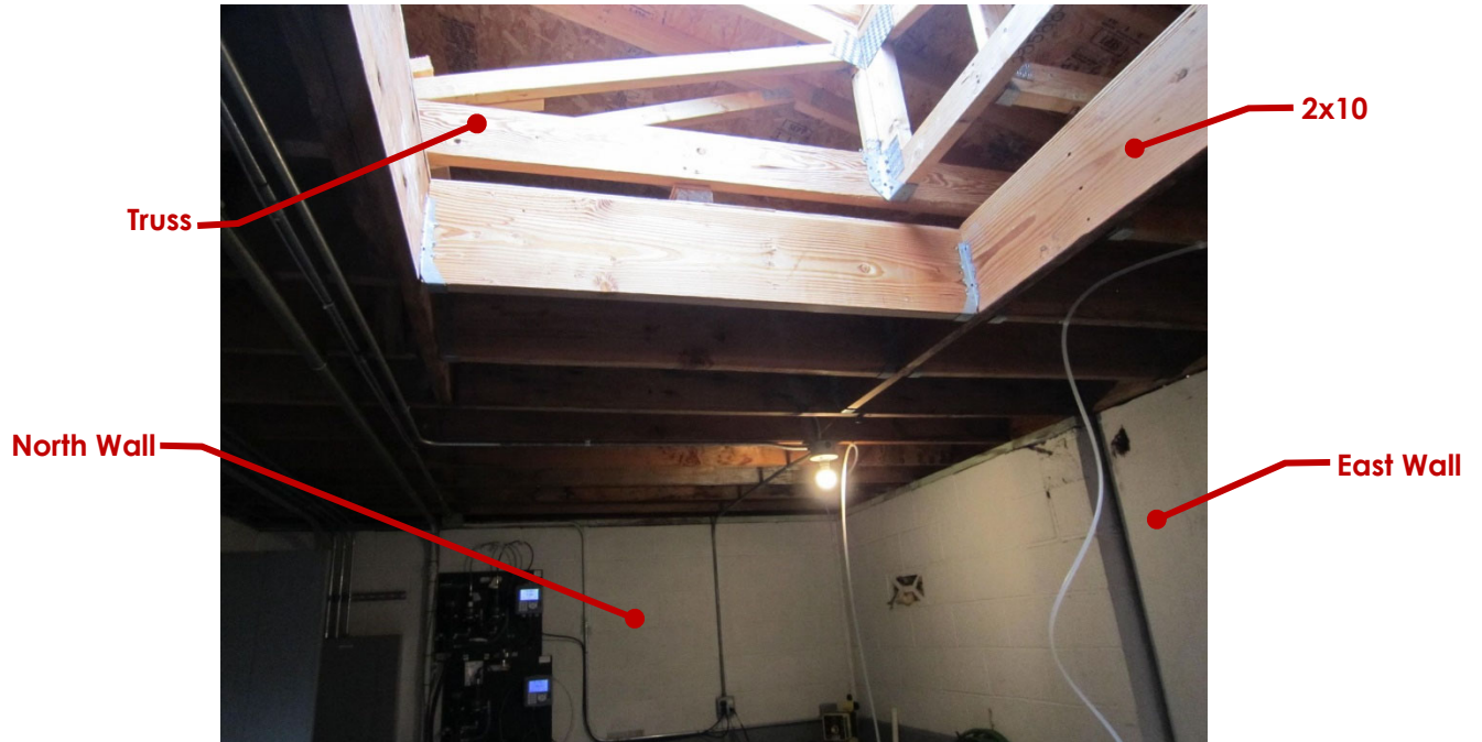
Photo 27 – Flow Meter Room (Looking North)
