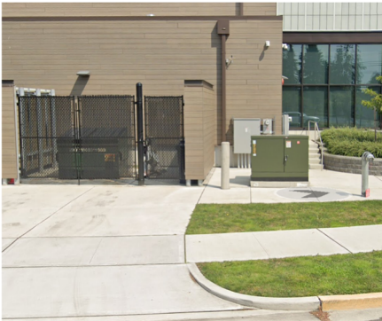
Roy H. Murphy Community Center Street-visible transformer and black vinyl-coated mesh utility/refuse yard gates.
