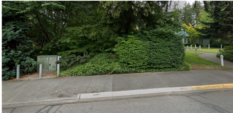
Fircrest City Administration Building Street-facing transformer located at the sidewalk edge.
