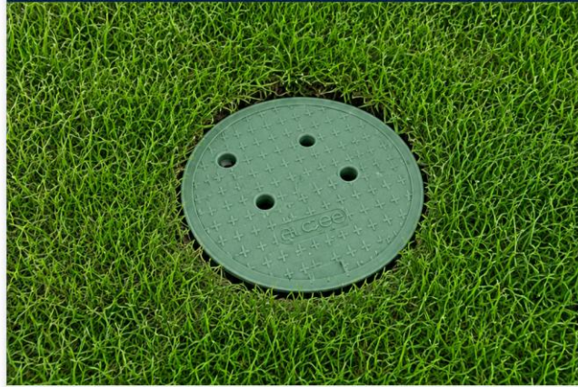
Fiber Access Point
